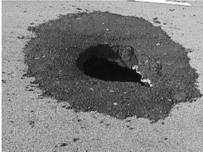
Fig. 1 - Veterans Highway Sinkhole Shortly Before Initial Patching
